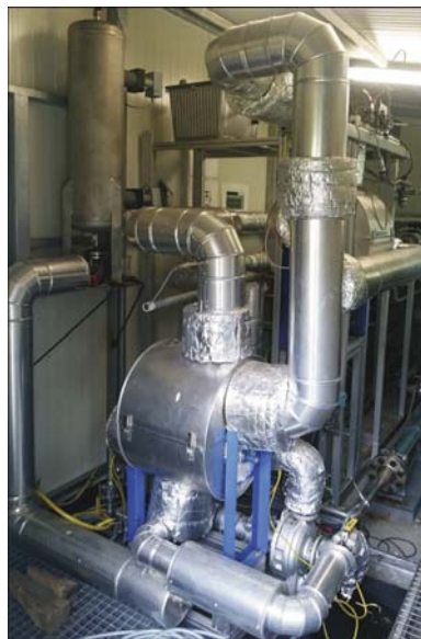
Fig. 3. CORC setup in a container that was placed outside of the laboratory due to safety reasons. Heat exchangers and piping system were thermally insulated with mineral wool.
